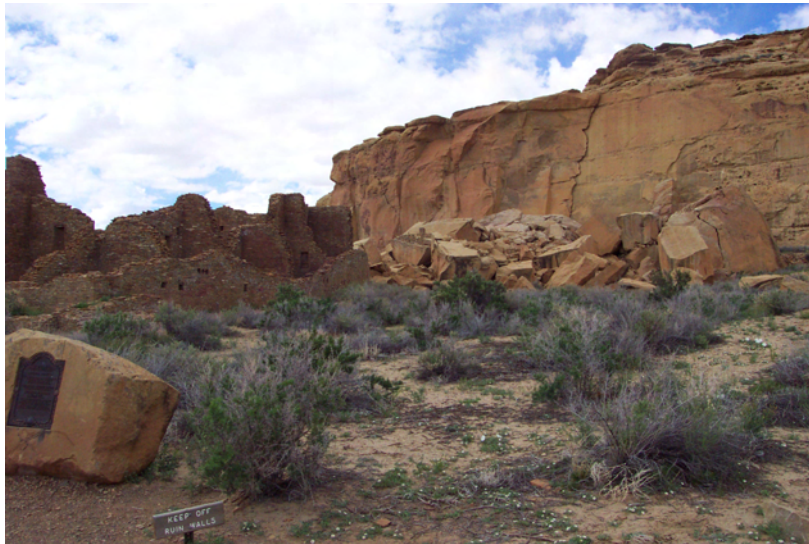
Pueblo Bonito showing rock fall from cliff face behind structure. (Photo courtesy of Dave Barz)
