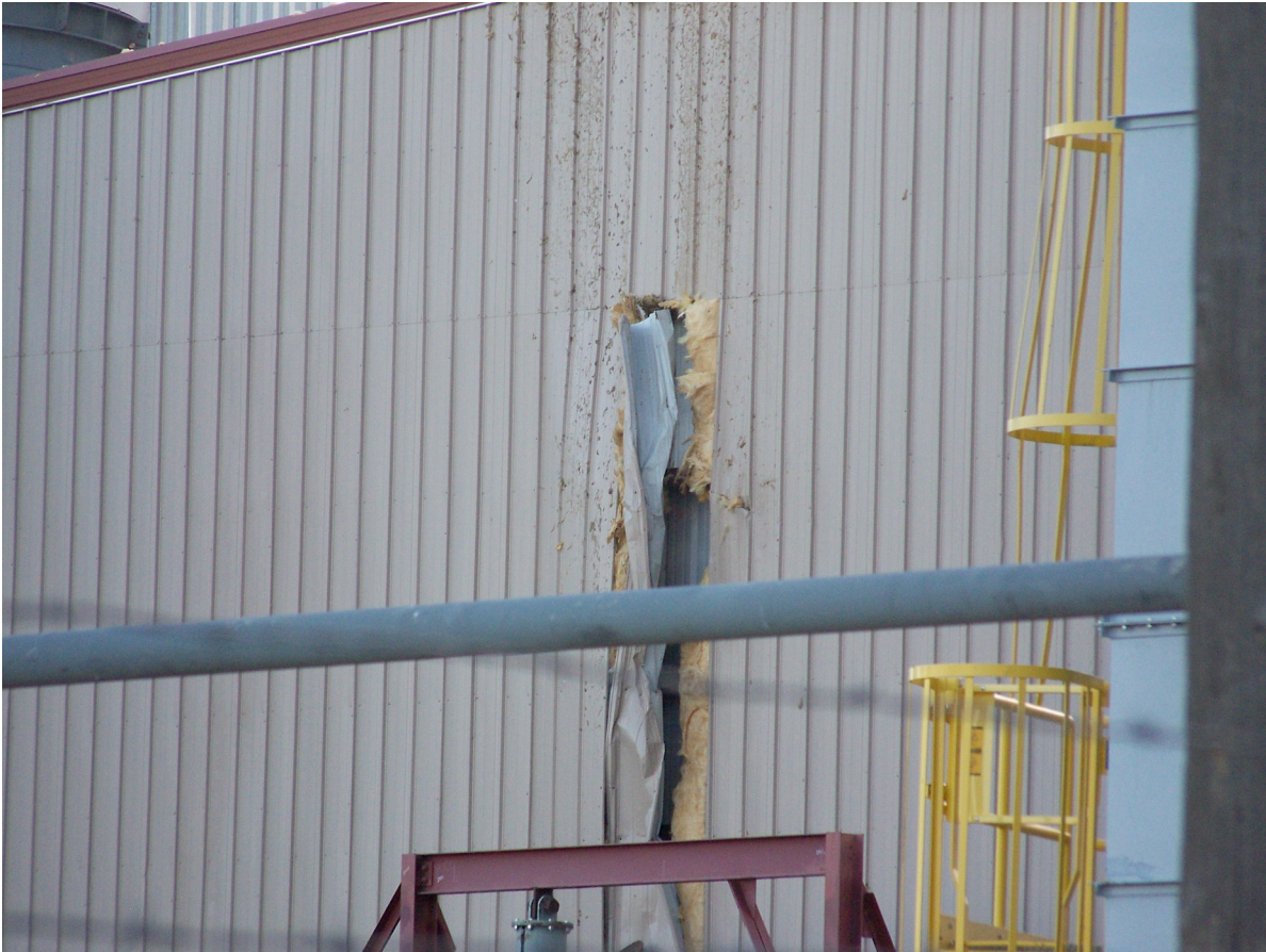
Picture of hole in wall of turbine housing at Lamar Light and Power coal-fired power plant, which was created on August 26, 2009 (photo taken by Shirley Warren on August 26, 2009).
